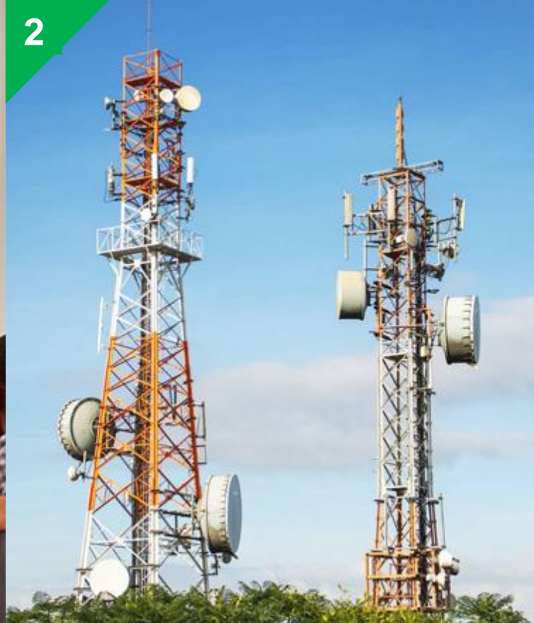
Turnkey Broadcast Station Equipment
